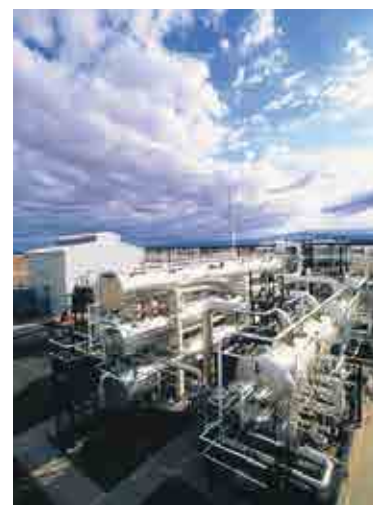
San Roque gas production facility in Neuquén (Argentina).
