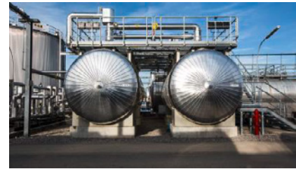
Wintershall has invested in recent years in the modernization of plant facilities.
