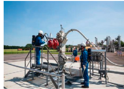
All the staff working at a production well at the natural gas production facility in Staffhorst wear special equipment such as respiratory masks.
