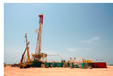
The Shuwaihat reservoir, which is situated in the western region of Abu Dhabi, lies partly under the mainland and partly under the sea of the Arabian Gulf.
