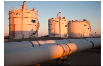
Wintershall export tanks at the Jakhira facility
