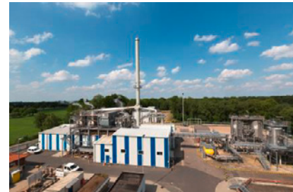
The steam flooding facility in Emlichheim produces hot steam, which makes the oil easier to extract from the reservoir.
